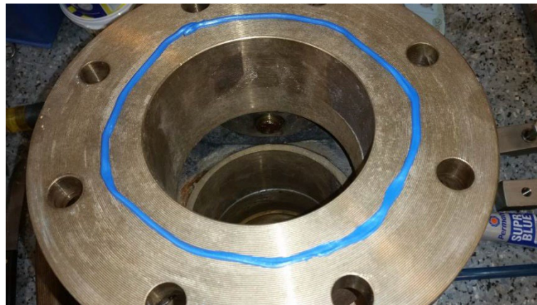
Figure 6. Sealing compound at the sea valve flange
